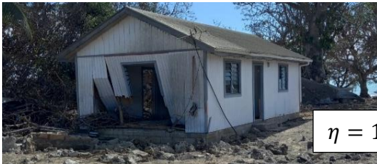
Fig. 1. Damages to the CRH at different inundation depths
